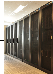
Remote data center
