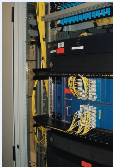
Apart from computing services, users may want to provision dedicated network services at the same time.
